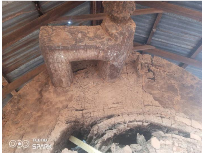
Plate. V: Dilapidation and termite invasion (Ikoro Obibie-Aku)
